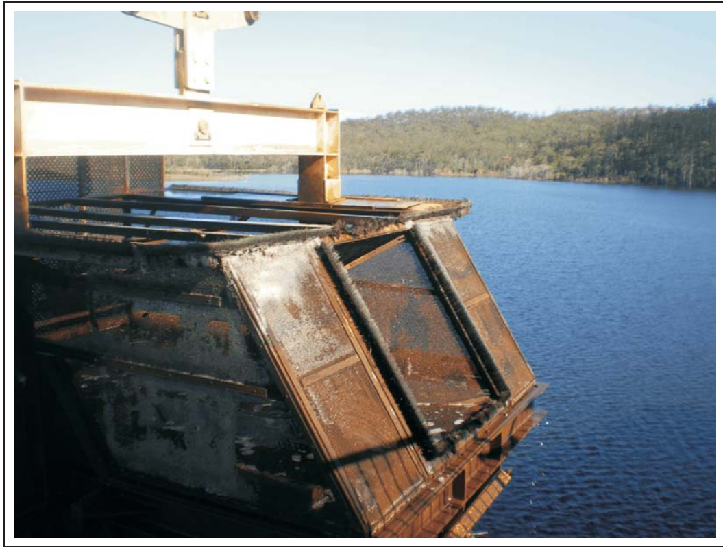
FIGURE 13(a) ENTRANCE TO UPSTREAM FISHWAY HOPPER
